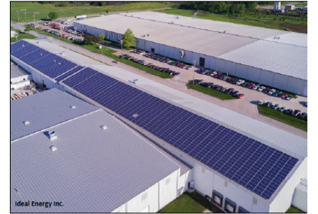
Iowa-based Agri-Industrial Plastics uses a 517-kilowatt roof-mounted solar array to provide a portion of its manufacturing power needs.
